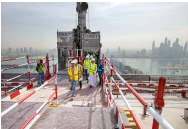
A rooftop tour, led by Aqil Kazim, Nakheel Chief Commercial Officer, of The Palm Tower construction site on 8 January 2019. Photo: © Nakheel
