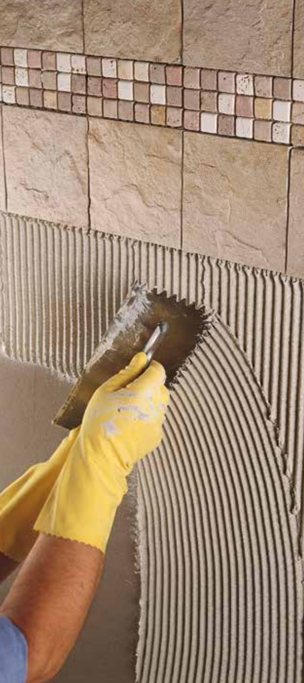
ADESILEX P9 was used to bond porcelain tiles on both horizontal and vertical surfaces.
